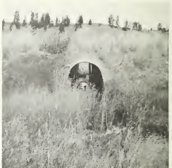
WEST ENTRANCE - Water in pipe
